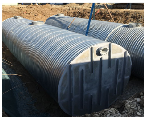
Fig. 7. Hydrocarbon separator with retention tank assembled at beneficiary
